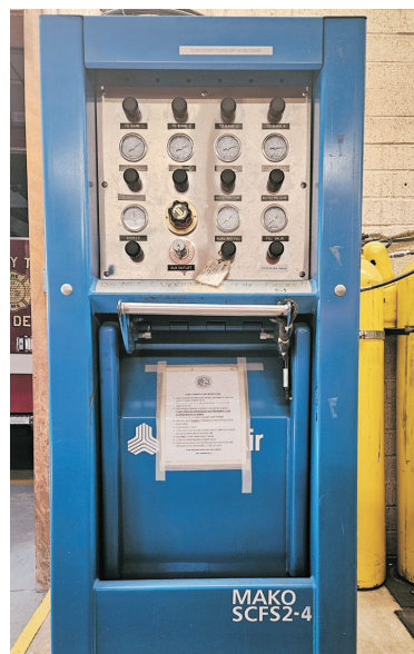
Stationary containment fill station
