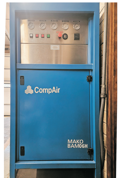
Breathing air compressor
